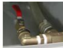
To drain the water in the boiler
